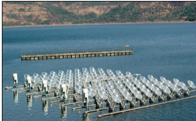
Fig. 4 Liquid Solar array, by Sunengy Pvt. Ltd.
