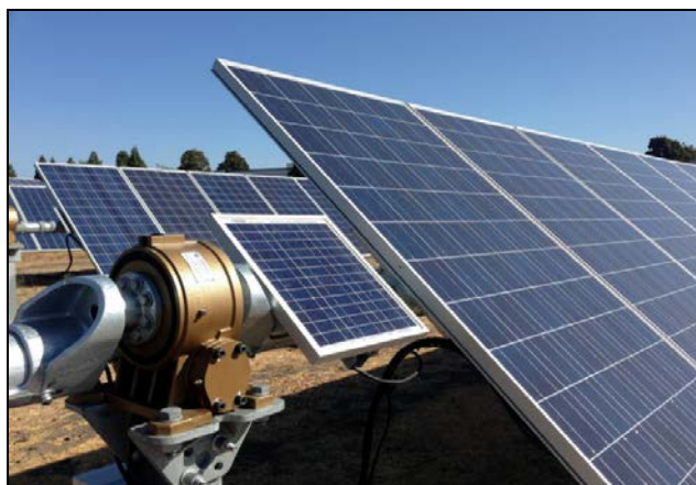
Fig. 8 Trackers for Solar Power Panels
